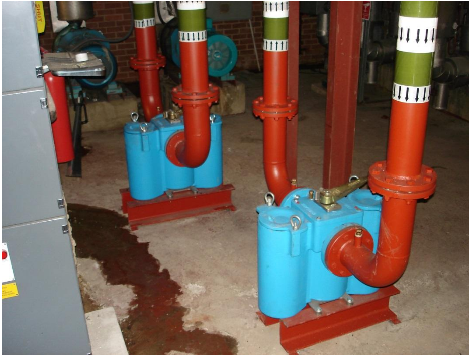
New duplex strainer units serving North West and South West fridge decks. The dirt collection baskets within each can be inspected and emptied without interrupting the flow to the fridges.
