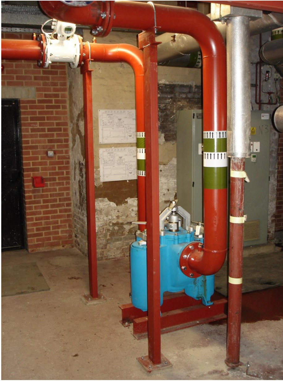
New duplex strainer and (top left) electronic flow meter serving Poultry Market. The flow meter is linked to the City's Building Management System, allowing the flow rate to be monitored and recorded continuously. There are separate meters for East and West Markets.
